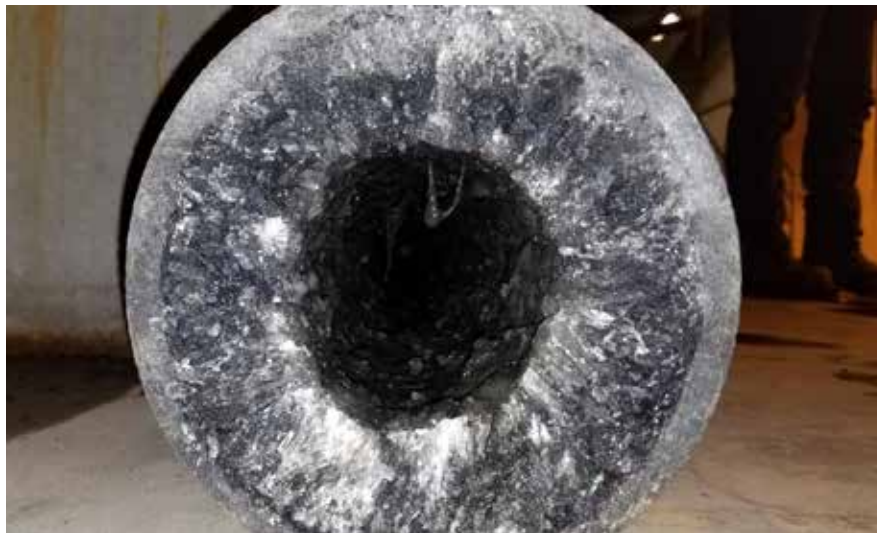
The Ocean County Utilities Authority (OCUA; Bayville, N.J.) excavated sections of solids transport pipe to discover a massive buildup of struvite.
