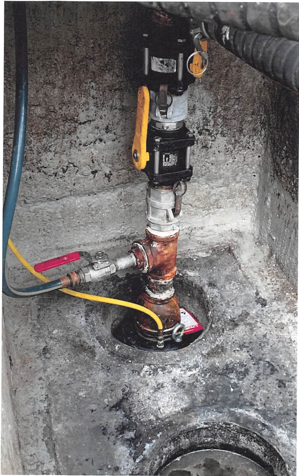
Struvite is a crystalline structure of magnesium, ammonium and phosphate that commonly builds up in pipe networks and is resistant to traditional maintenance methods for removal.
